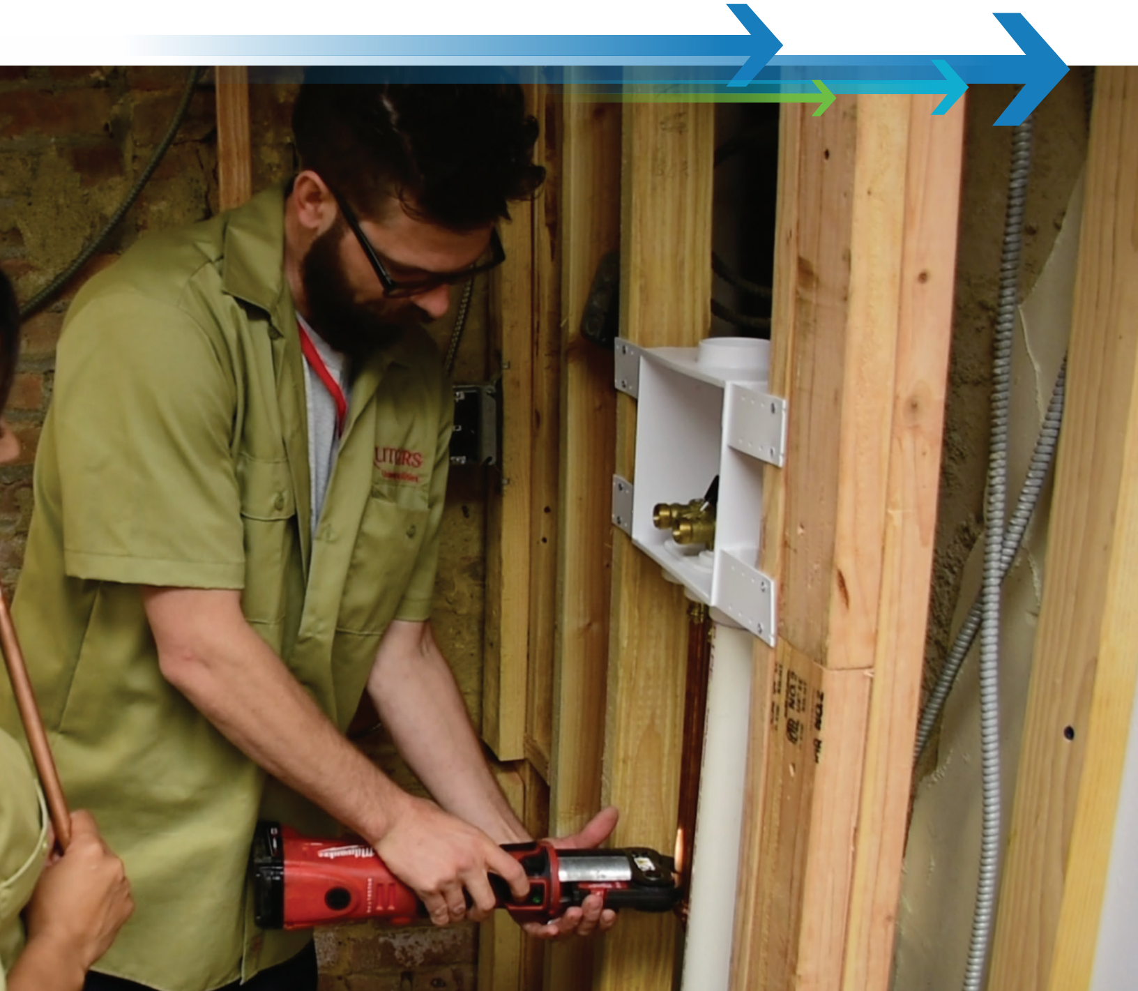
Najia Boumahdi (left) gets on-the-job training from Senior Pumber and Maintanance Mechnic Roman Duffy, as part of the Craft Trainee Program.
